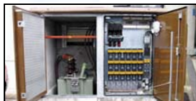
The transformer and L.V. compartments
