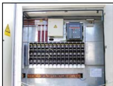
L.V. distribution panel
