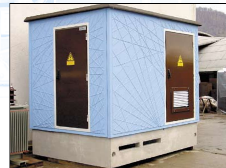
Concrete walk-in unit substation BK003I
