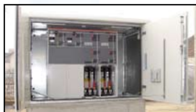
M.V. compartment fitted with RMU
