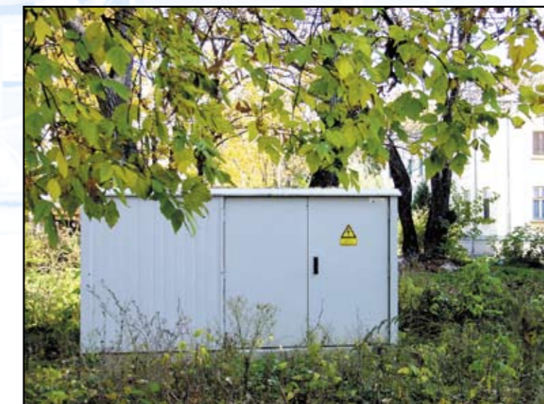
SIK 35-23 Metal insulated packaged unit substation mounted and operational
