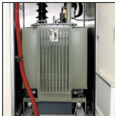
The transformer fitted with wheels
