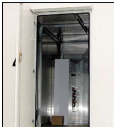
Metal insulated walk-in unit substation
