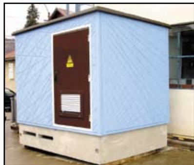
Concrete walk-in unit substation
