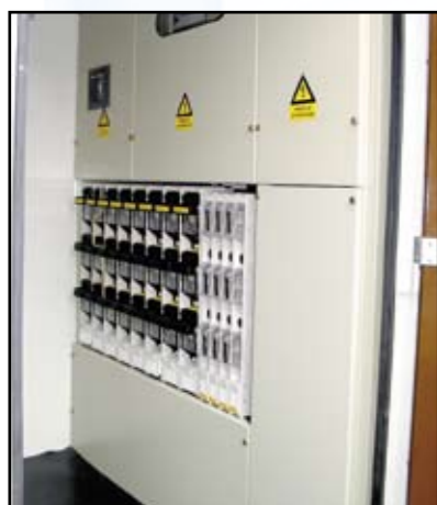
L.V. distribution panel fitted fuse switches
