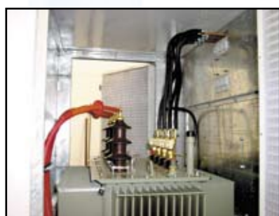
The transformer compartment
