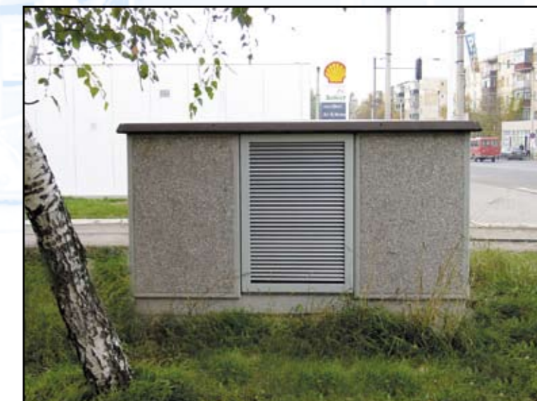
Concrete packaged substation BK 003 installed and operational
